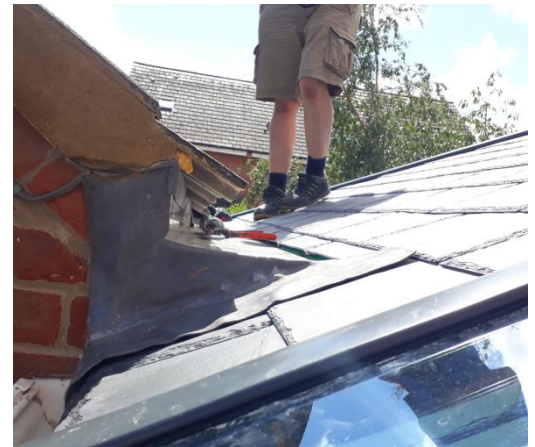
Partial tapered box gutter with garage roof cut away. Check frame height and maximum height of the tapered box gutter in this situation.
